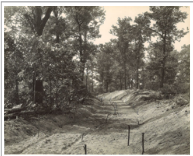
A 1928 picture of Roundhill alley being staked out for construction (from the Sheridan Library archive).
